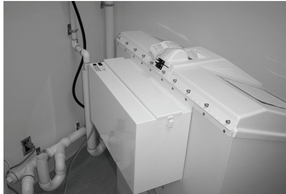
Figure 1. GUS® Model G14SD Vapor Management System Installed on Olympus DSD
